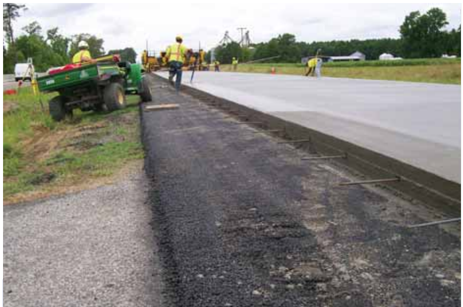
In the unbonded section, they used tie bars to tie the two lanes together and tie the shoulders to the lanes but no reinforcing steel was used.
