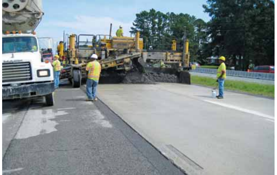
After repairing any broken concrete, the contractor used a stringless, laser-guided system to measure the profile of the old pavement and place the bonded overlay.
